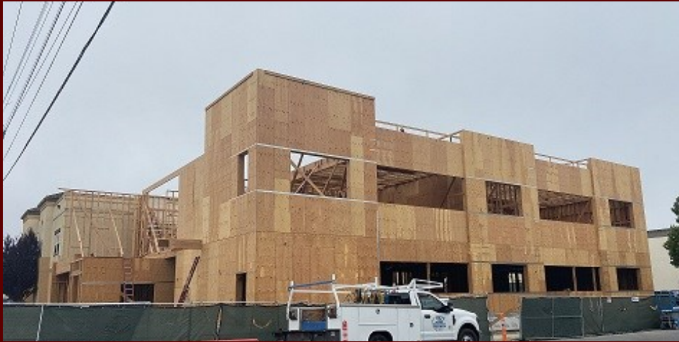
KING CITY—NEW EXPANSION COVERED WITH SHEER WALL ANTICIPATING INSTALLATION OF THE WINDOWS
