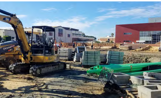
Work continues on the Main Campus central plaza in this January 2020 photo.
